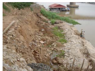
Fig.3b Collapse of retaining wall
