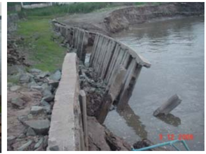
Fig.4b Collapse of wall (view from river)
