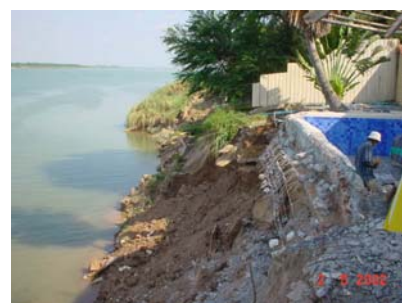
Fig.2 Collapsed natural slope
