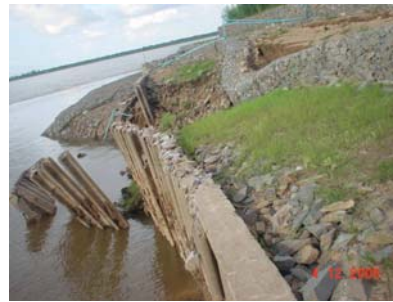
Fig.4c Collapse of wall (view from side)
