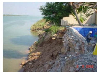
Fig.2 Collapsed natural slope
