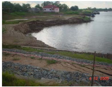
Fig.4a Slope erosion
