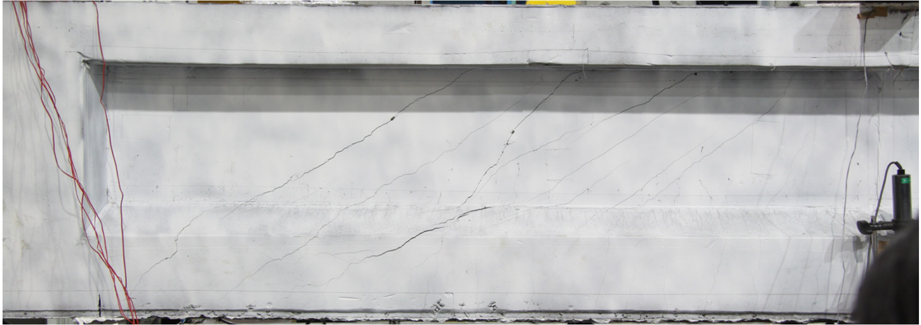
Crack pattern at the peak load: C-s300-II
