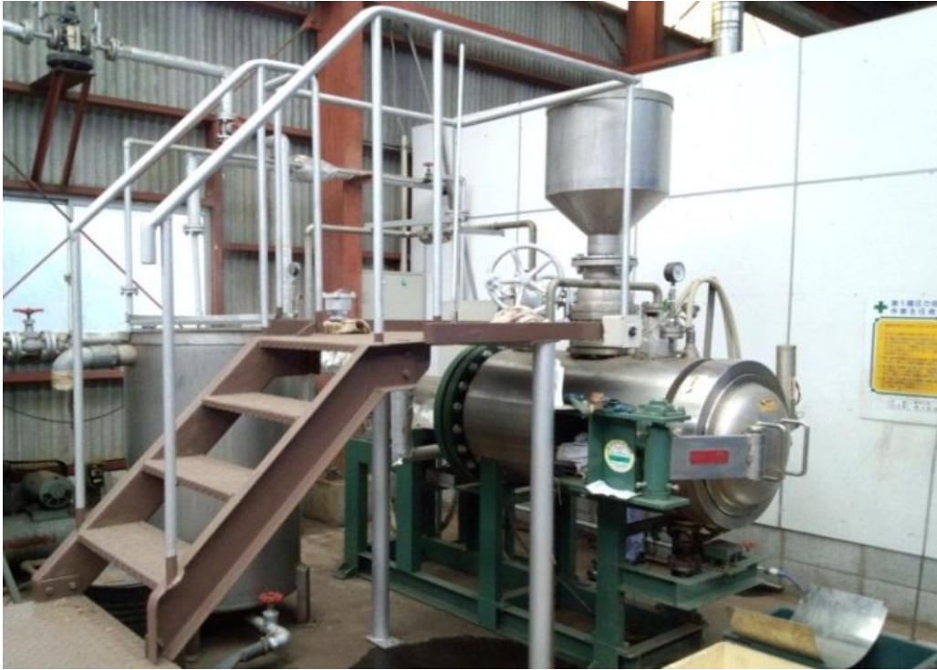
Fig.4.2. Snapshot of the HTT facility
