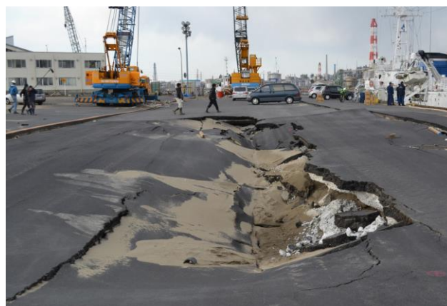
Figure 1.3. Depression behind quay wall at Kashima port (EERI, 2011).
