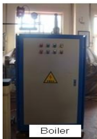
Fig. 2.2 The electric steam boiler used in the hydrothermal treatment
