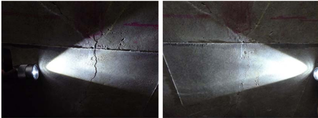
(a) Light from the span center (b) Light from the hunch side → Same crack is shoot, but shade appears only in (a) because of the gap.
