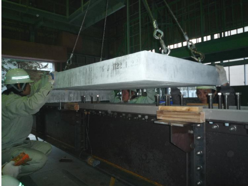
(a) Settlement of pre-cast concrete deck
