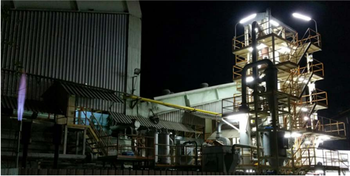
Figure C1: The photograph of 650 kW th fluidized bed gasification facility at Siam Refractory Industry Co.Ltd. (SRIC), Thailand
