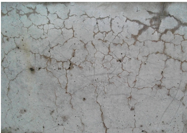
Fig. 1.2 Crack in concrete
