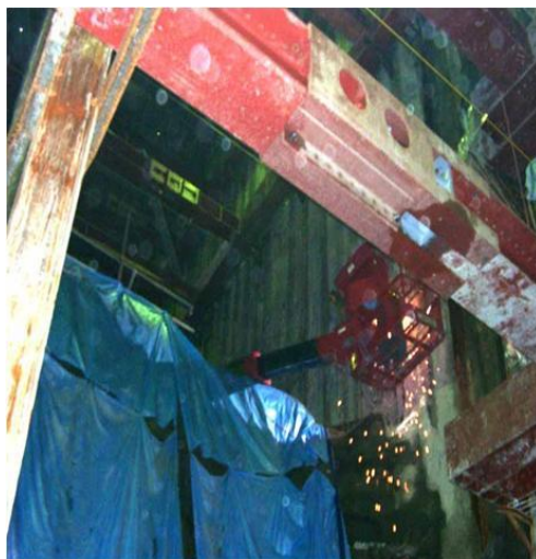
写真 3.23 溶接火花の飛散状況
