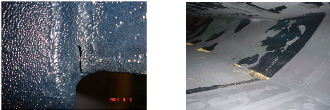
Fig. 1.15 FAC in moisture separator reheater
