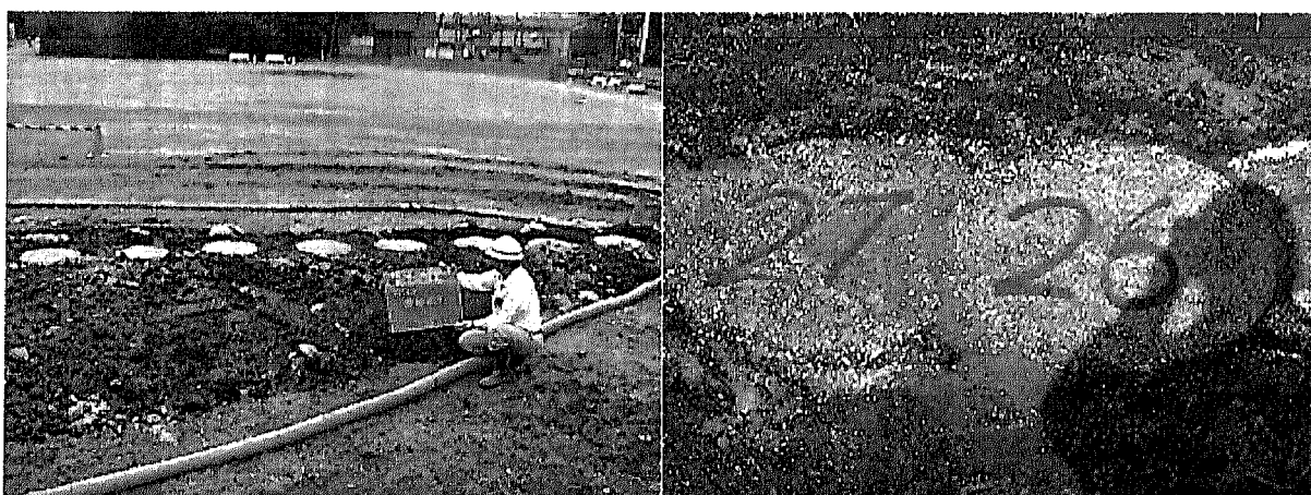
(a) Condition before overlapping of the column (b) Overlap each improvement column
