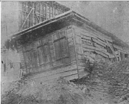
(g) A collapsed house at Tekirdag, build of wood on top of bricks.
