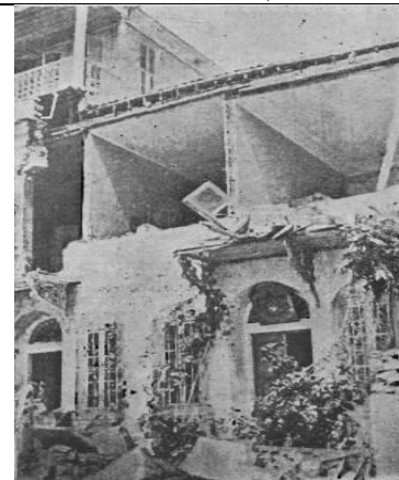
(h) Damaged building at Canakkale (Sadi, 1912).
