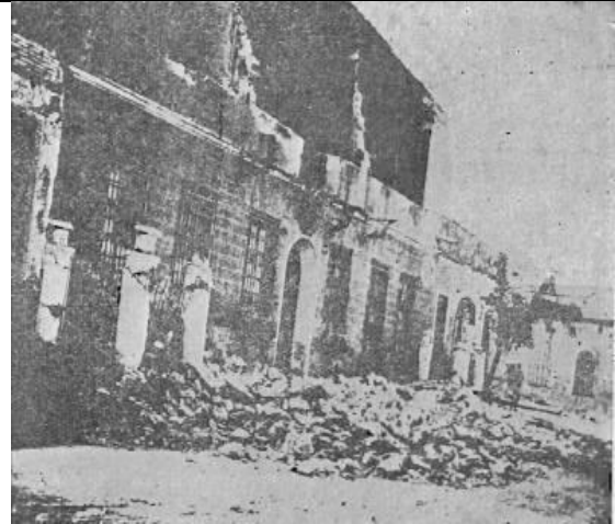
(f) The palace of the Austro-Hungarian Empire consulate was partly damaged (Gelibolu-Canakkale; Mihailovic, 1933).
