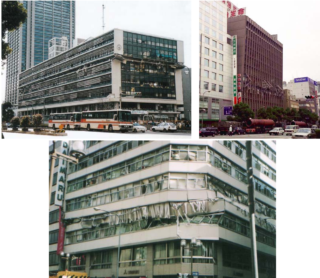
Fig 1.3 Mid-level collapse observed in Great Hanshin earthquake 1995
