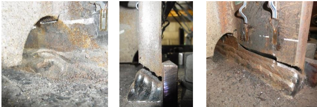
(a) Crack at the weld access hole (b) Crack at the weld toe (c) Propagation of cracks
