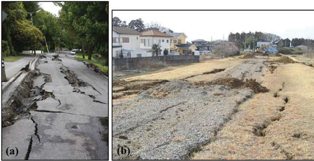
Figure 4.16. Damages induced by lateral spreading; (a) 2011 Christchurch earthquake, (b) 2011 Tohoku earthquake (Towhata, 2011).
