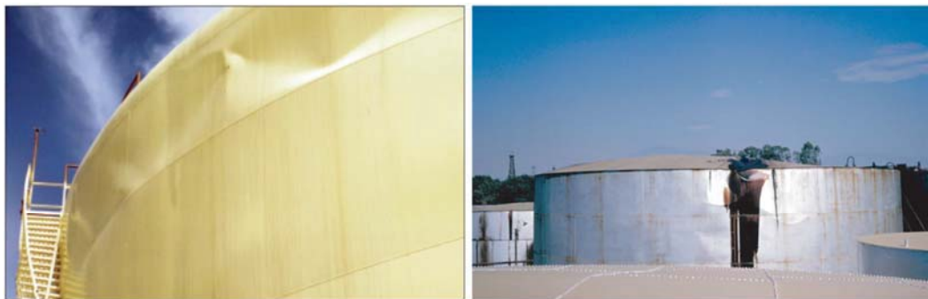
Upper shell of tank suffered damage by sloshing.
