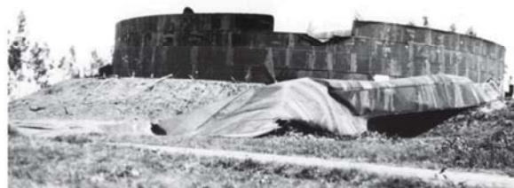
The tank lost its roof and a portion of upper shell during 1933 Long Beach, California earthquake.
