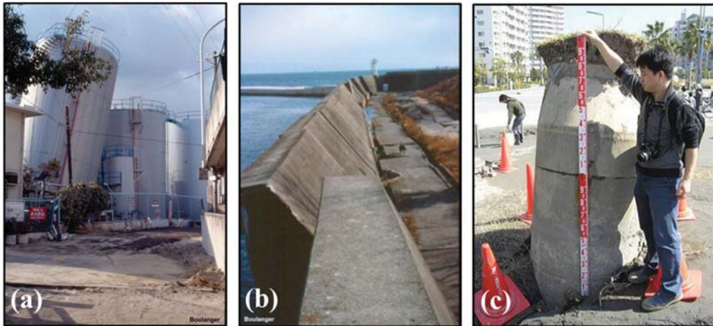
Figure 4.14. Soil liquefaction damages; (a) Tank overturning in 1995 Kobe earthquake (UC Davis website), (b) Quay wall overturning in 1995 Kobe earthquake (UC Davis website), (c) Buried structures flotation in 2011 Tohoku earthquake (Towhata, 2011).
