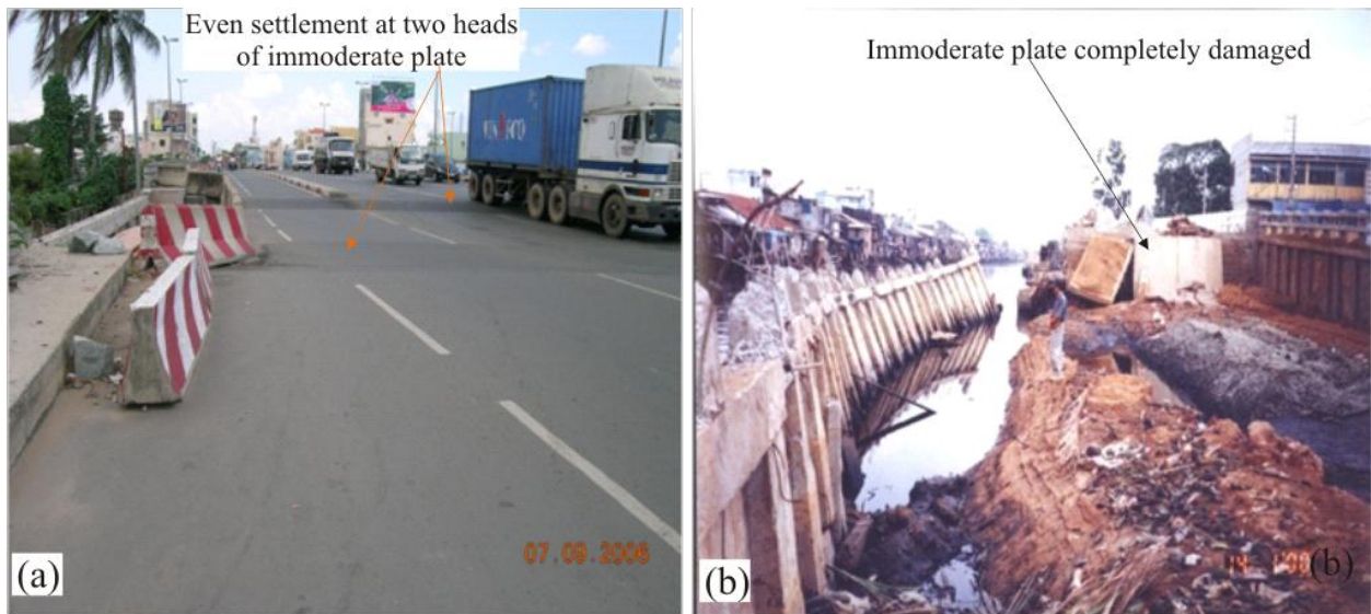
Fig. 1.7. (a) Even settlement at two heads of immoderate plate of Vanthanh Bridge in district 1 (b) Approach and immoderate plate of bridge in district 8 Hochiminh City suddenly collapsed and completely damaged.
