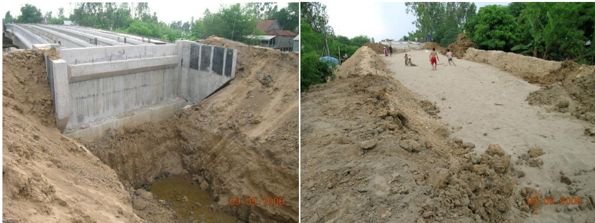
Fig. 1.8. Contiguous zone of bridge propped by piles and embankment building in Dongthap province MD.
