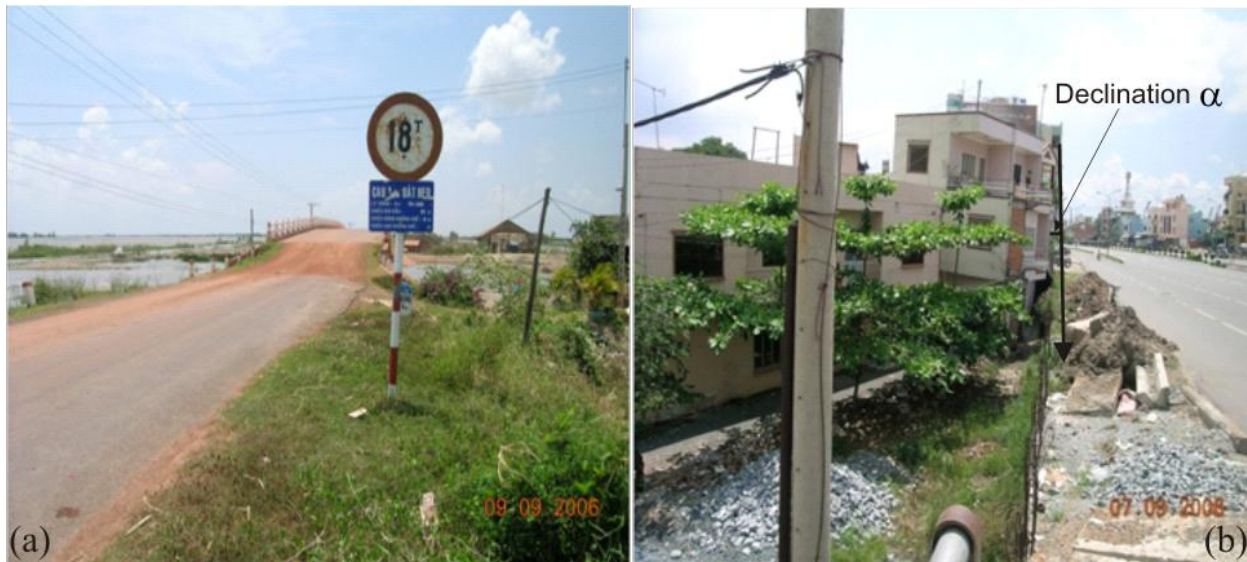
Fig. 1.6 . (a) Settlement of approach of bridge in Dongthap MRD; (b) Settlement of approach of Vanthanh Bridge made house be declinational and damaged in district 1 Hochiminh city.
