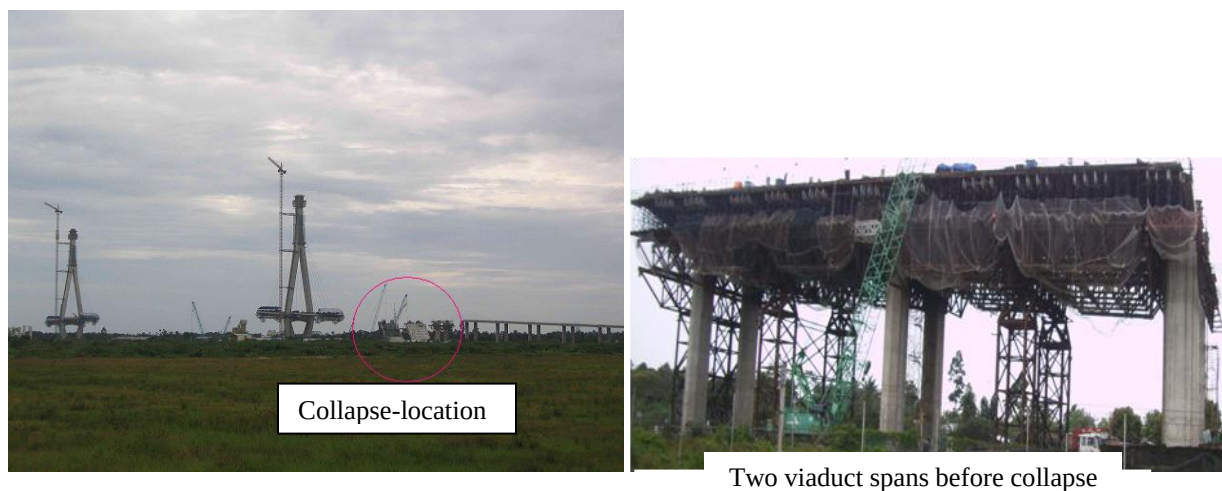
Fig. 1.4. Location of collapsed viaduct spans at Cantho Bridge construction site on Sep. 26, 2007.
