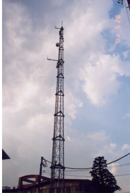
Figure 2.5: Urban observation tower for urban climate analysis located in Tokyo suburban area in Kugahara. Picture taken from http://www.ide.titech.ac.jp/~kandalab/
