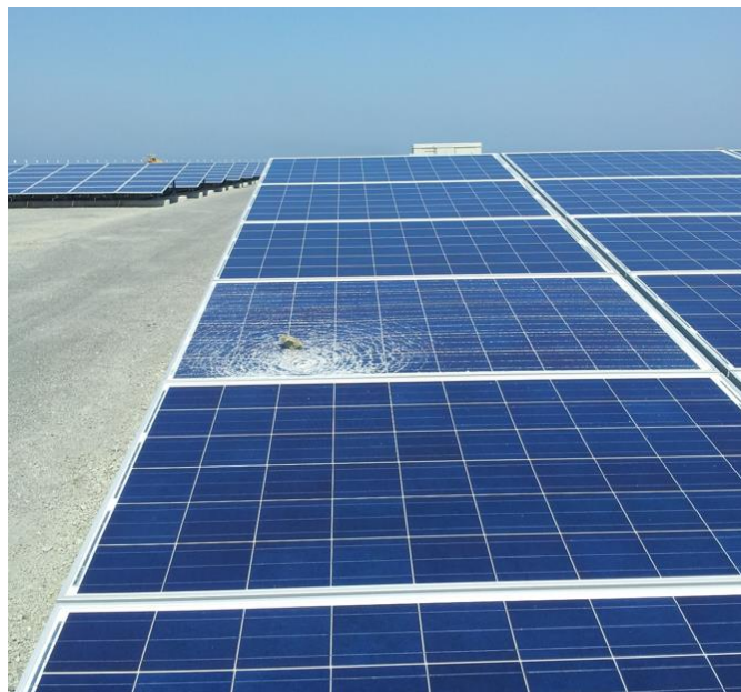
(b) Detected Glass breakage (pattern1: broken wire)
