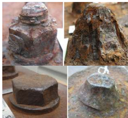
Figure 1.3 Corrosion in a bolted connection [31]
