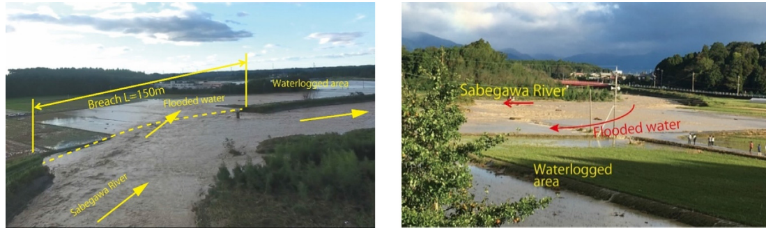
Fig. 22. Breached point on Sabigawa River (in Naka River system) in Kita-owagu area, Otawara City, Tochigi Prefecture. Left photo: View from upstream side, Right photo: View from left levee (Photos provided by Tochigi Prefectural Office with English translation).
