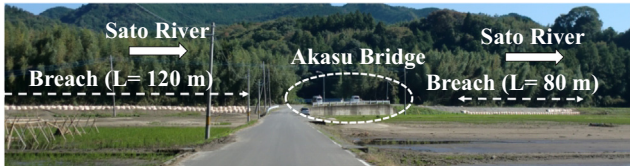
Fig. 30. Temporary restoration works of right levee of Sato River at Point C in Fig. 29 (near Akasu Bridge).
