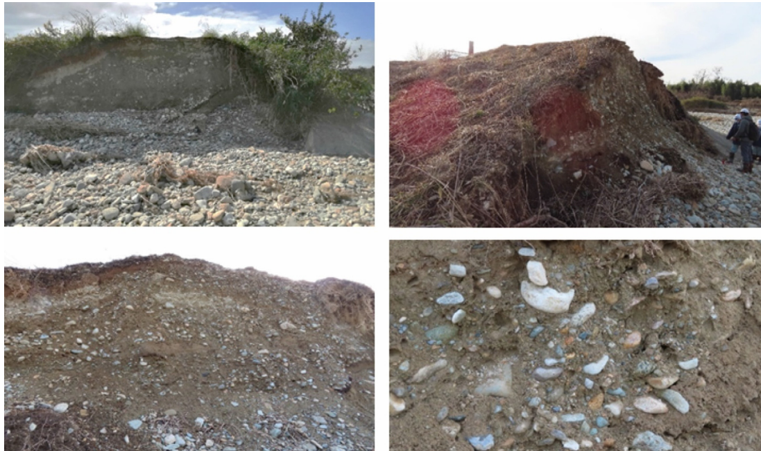
Fig. 25. Damage to levee at breach point. The embankment contains many boulders along with the soil. The embankment was presumably constructed from the surrounding sediment (Photos taken by Unno on December 2, 2019).
