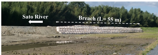
Fig. 32. Temporary restoration works of left levee of Sato River at Point D in Fig. 29.
