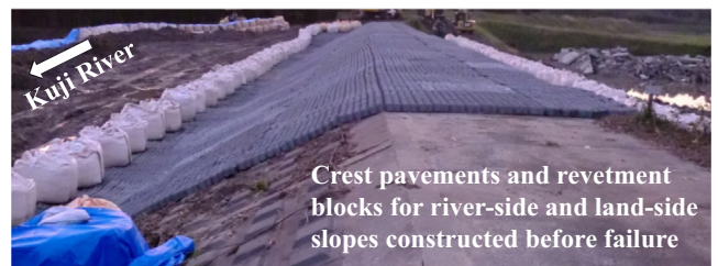
Fig. 28. Crest pavements and revetment blocks for river-side and land-side slopes constructed before failure at 34.0 k of the Kuji River.
