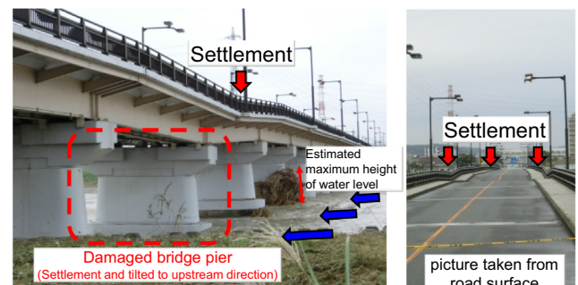
Fig. 41. Damaged river bridge pier caused by scour.
