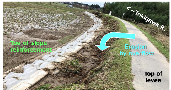
Fig. 11. Levee that survived erosion by overflow.
