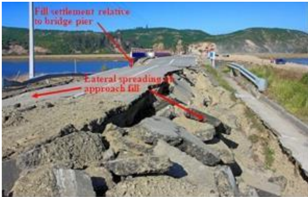
Figure 2.1.3 Lateral spreading at Raqui 2 bridge during 2010 Maule Earthquake in Chile (Yen et al, 2011)
