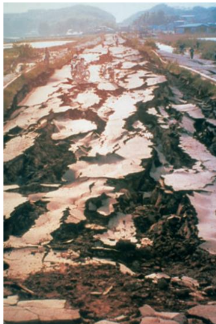
Figure 2.2.1 Damage to road embankment during the 1964 Niigata Earthquake (Hamada et al. , 1986)
