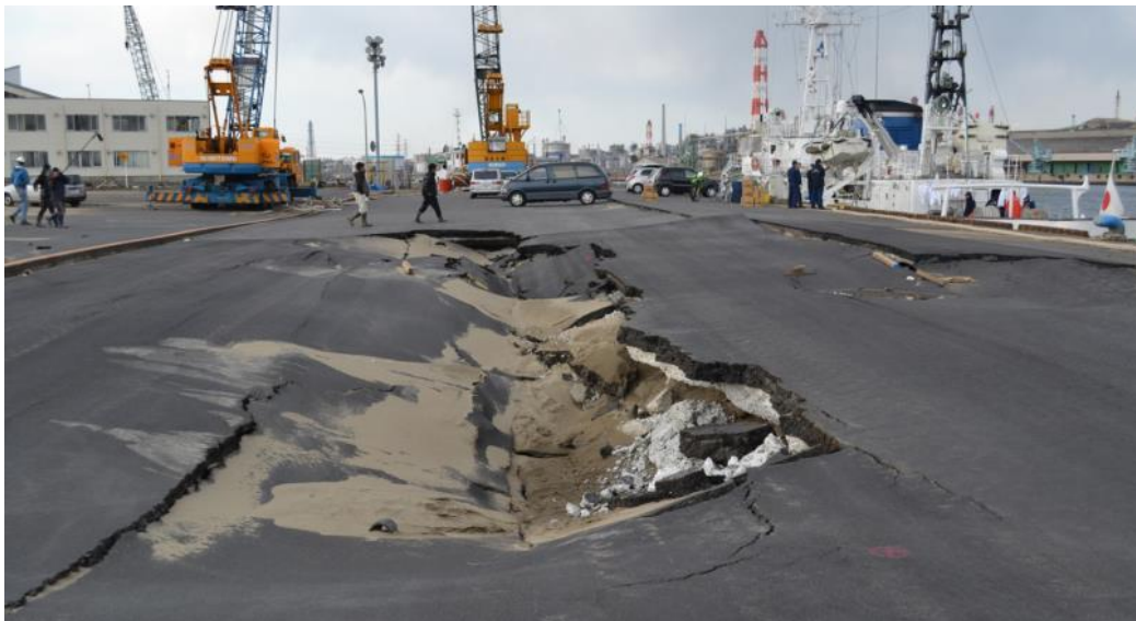
Figure 2.1.4 Depression behind quay wall at Kashima port (EERI, 2011)
