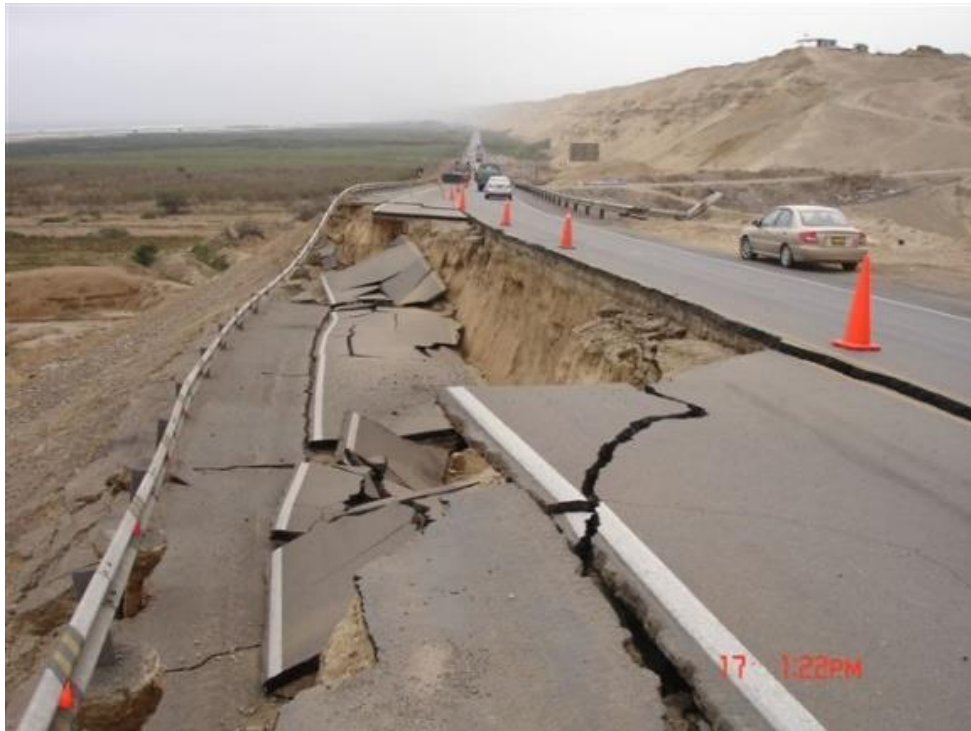
Figure 2.1.2 Embankment failure due to liquefaction on the Pan-American Highway during 2007 Peru earthquake (MCEER, 2007)
