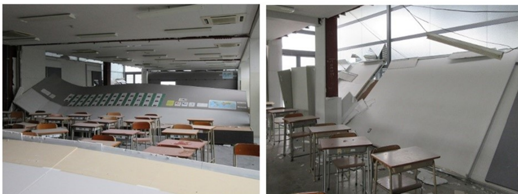
Fig. 1-1. Damage of non-structural LGS wall during Kumamoto earthquake[1-4].
