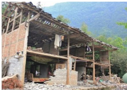
Fig. 1-2. Damage to masonry-infilled timber frame after 2013 Lushan earthquake in China[1-18].
