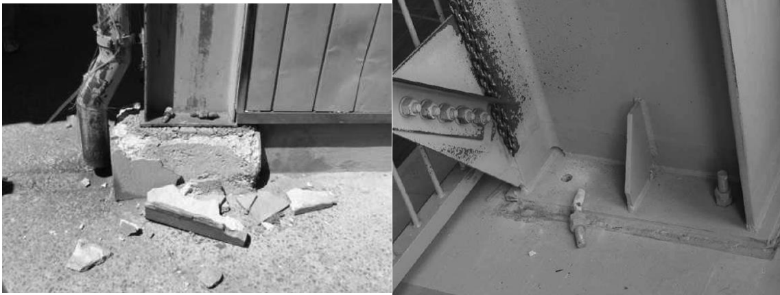
Photo 1-1 Anchor rods fracture in 2011 Tohoku earthquake [1-2]
