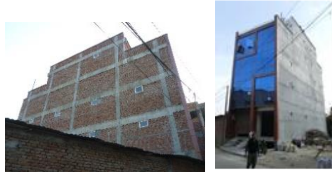
a) Southeast view b) Northeast view Fig. 2 - Overview of the target building
