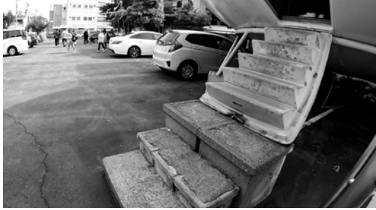
Fig.2. Foundations are on the concrete legs which were not included in the original concept and additional stairs were needed in order to be able to come inside a house. The blue upper stairs are made of plastic with metal elements for joints, and originally were automatic and controlled by buttons inside a house
