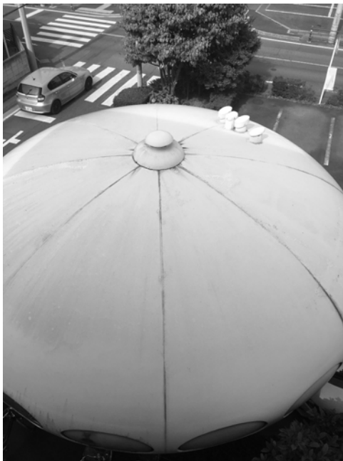
Fig.6. Stains of corrosion can be seen on the roof but no water leakages or cracks in the structure were reported to date
