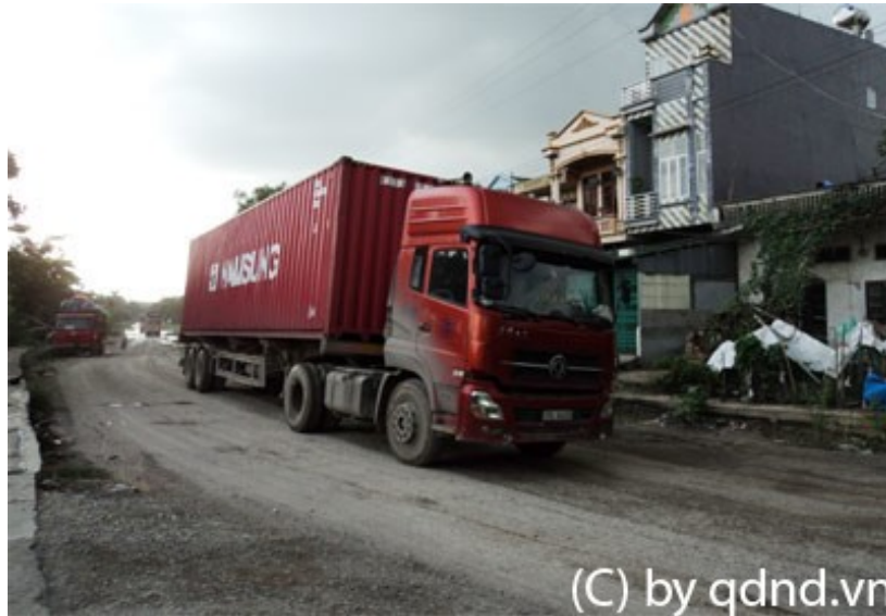
Fig. 1.1 A damaged road because of overload trucks
