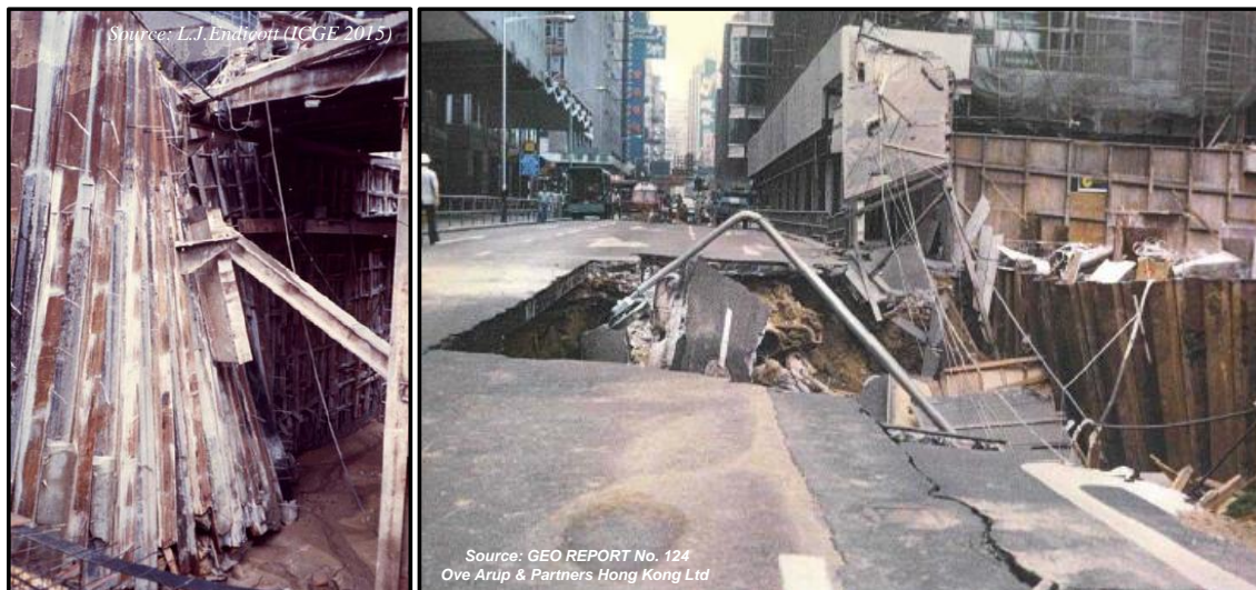
Figure 2.11: Sheet pile failure and Queen's Road collapse during Edinburgh Tower basement construction
