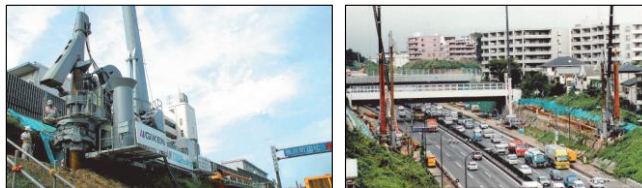
Construction of cantilever type embedded retaining wall in a narrow space adjacent to the highway with operation (Yokohama, Japan)
