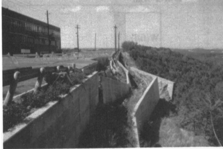
Figure 2.12: Failed section of retaining wall.
