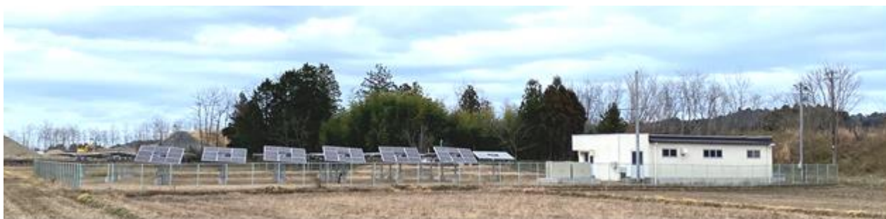
Fig.1.5 Solar panel in Fukushima
