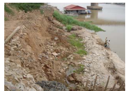
Fig.3b Collapse of retaining wall
