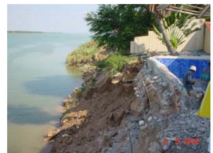
Fig.2 Collapsed natural slope
