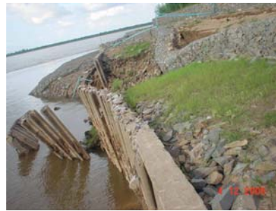
Fig.4c Collapse of wall (view from side)
