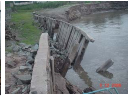
Fig.4b Collapse of wall (view from river)
