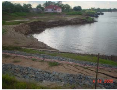
Fig.4a Slope erosion
