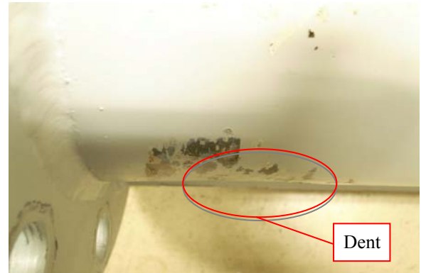
Fig. 10 Dent on the Pipe
