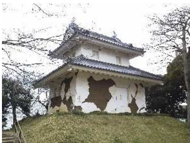
Figure 1. A historical building damaged by the earthquake. Tsuchiura castle, Ibaraki prefecture. Photo courtesy of T. Kimoto.
