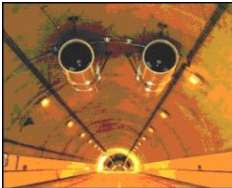
Fig. 1.29 Jet fan for tunnel ventilation system (1.48) .
