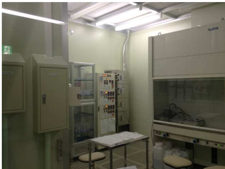
Fig. 3.2: Image of the thermal oxication system
