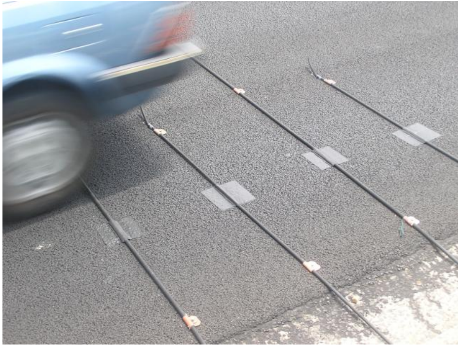
Figure 2.4: Pneumatic traffic detection systems (TCS for Surveys, 2013)
