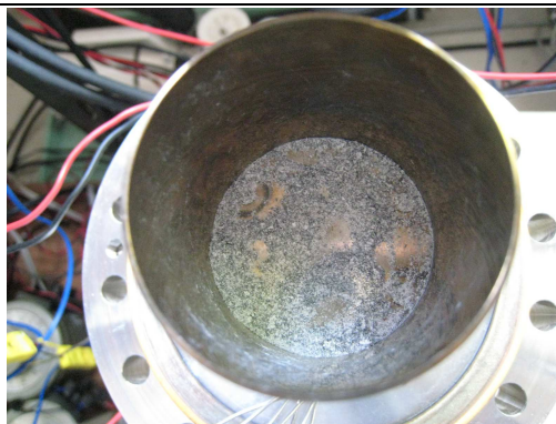
Fig.3.21 material accumulation on the bottom
