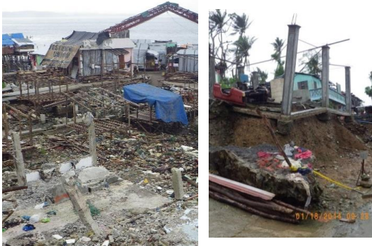
Fig. 10. Typical damage along the coast south of Tacloban Airport (left), and along the coast of downtown Tacloban (right). In both locations, waves were present.
