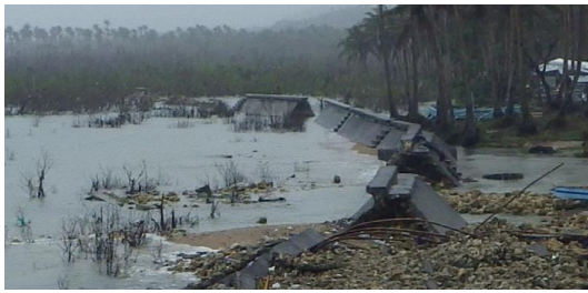
Fig. 13. Damage to the coral-fill Hernani seawall.
