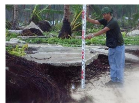
Fig. 12. Damage to a concrete foundation near the Guiuan PAGASA station.
