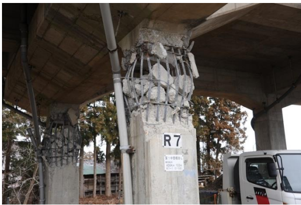
(a) Flexural shear failure of columns.
