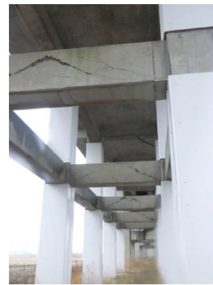
(b) Shear cracking.
