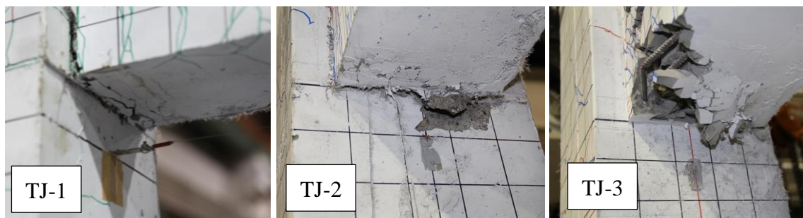
Photo 5.4.4 Damage at the bottom of the beam by the end of tests.
