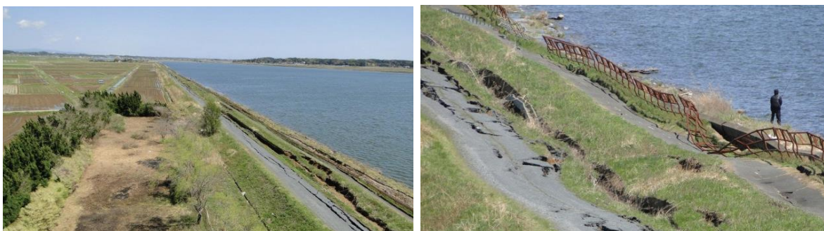
Figure 1.8. Views of slumped Hinuma River Levee and cracks induced by liquefaction (GEER, 2011).
