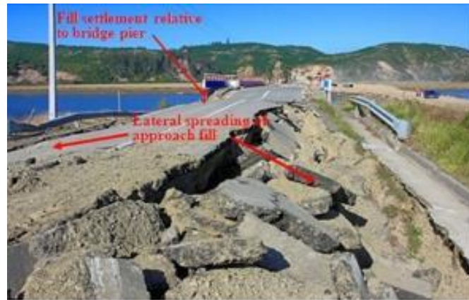
Figure 1.6. Lateral spreading at Raqui 2 bridge during 2010 Maule Earthquake in Chile (Yen et.al 2011).
