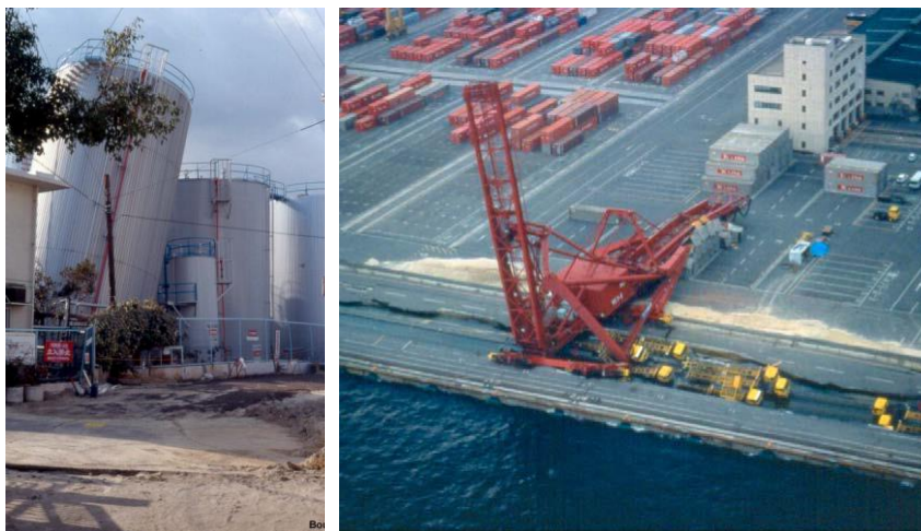
Figure 1.5. Tilting of gas tank and damage to port facilities during 1995 Kobe earthquake (University of Washington, 2000).
