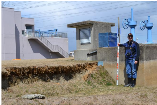
Figure 1.4. Liquefaction induced differential movements around buried tanks of a water treatment plant in Kashima City during 2011 Great East Japan Earthquake (EERI, 2011).
