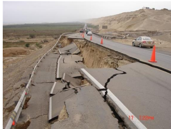
Figure 1.7. Embankment failure due to liquefaction on the Pan-American Highway during 2007 Peru earthquake (MCEER, 2007).
