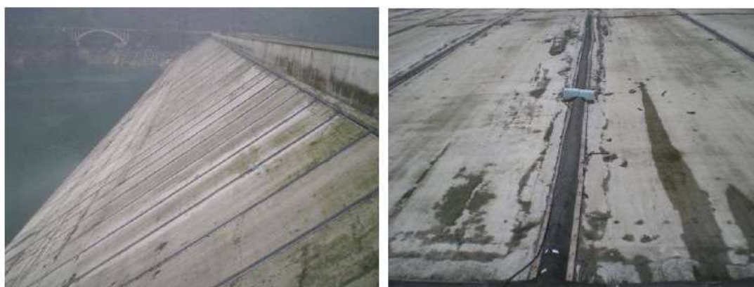
図-2.4.24 Concrete face of Zipingpu CFRD after repair: view of upstream face (left) and detail of vertical joint (right) 34)
