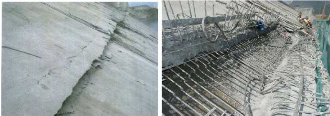
図-2.4.26 Damage of concrete face of Zipingpu CFRD: damage at longitudinal joint (left) and repair of longitudinal joint (right) (Photographs courtesy Xu Zeping, China) 34)
