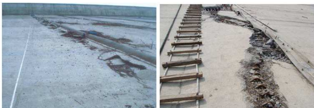
図-2.4.25 Damage of vertical joint of concrete face of Zipingpu CFRD (looking towards crest)(left): preparation of repair works along vertical joint (right)(Photographs courtesy Xu Zeping. China) 34)
