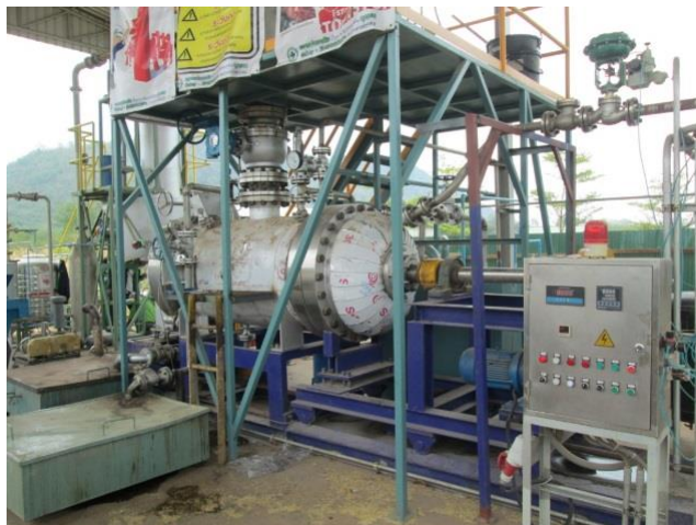
Figure 2-5 Hydrothermal pilot plant (Courtesy of SCG)
