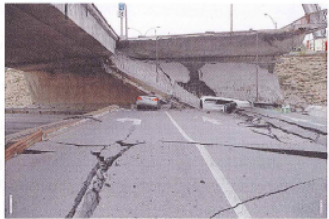
Fig. 1.3 Failure of concrete bridge 11)
