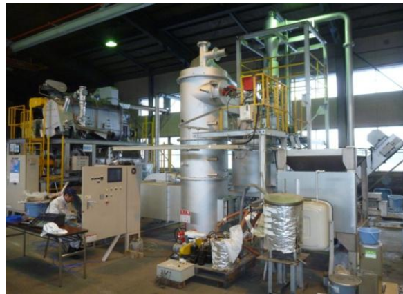
Figure 1-2 Photo of the pilot-scale gasification plant
