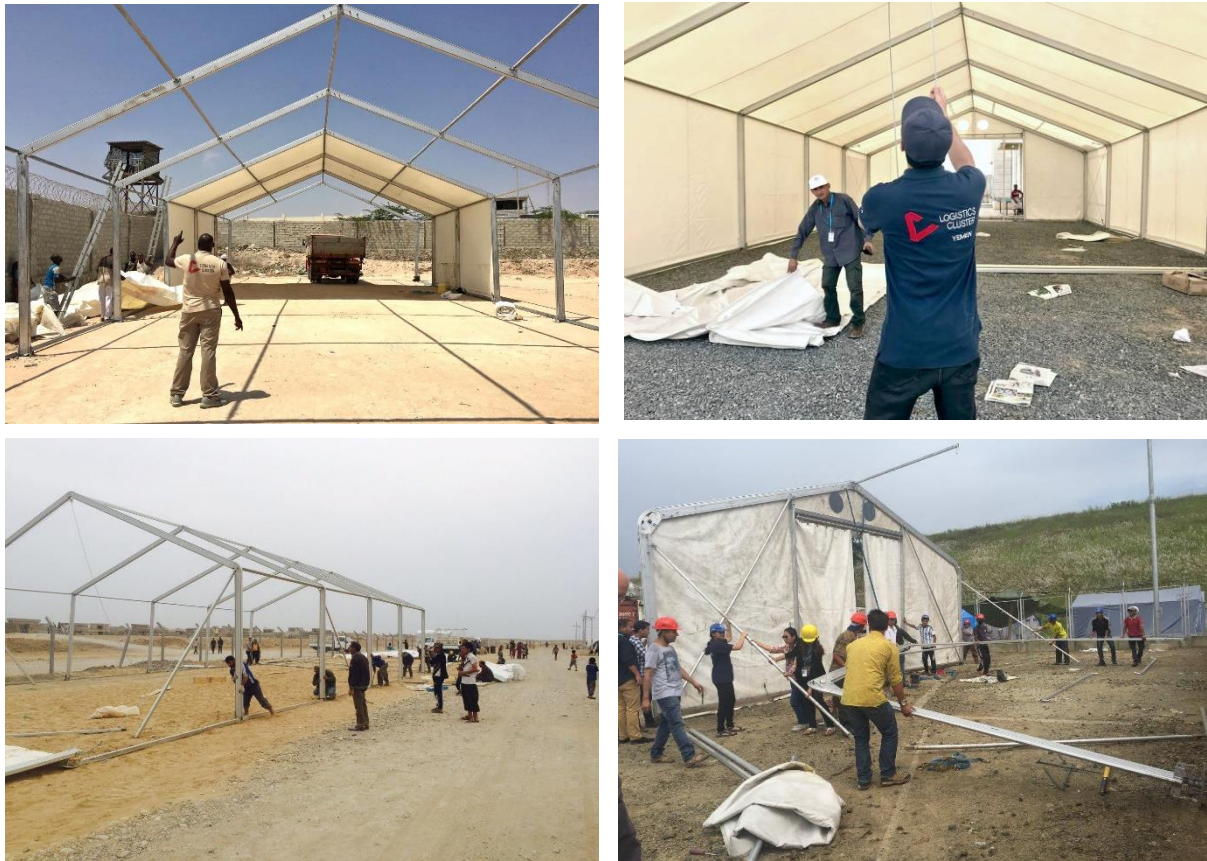
Figure 1.7: Setup of mobile storage units
