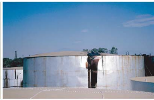
The roof and roof-shell junction suffered damage during 1952 Kern County, California earthquake.
