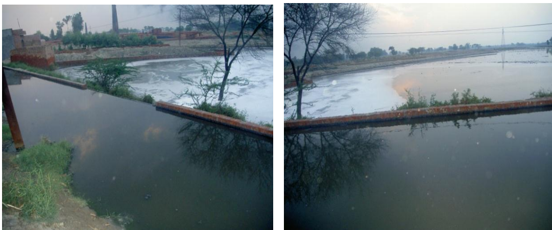
Fig. 4.12: Drain 3 overflow situation observed in 2011 (Picture taken in April 2011)
