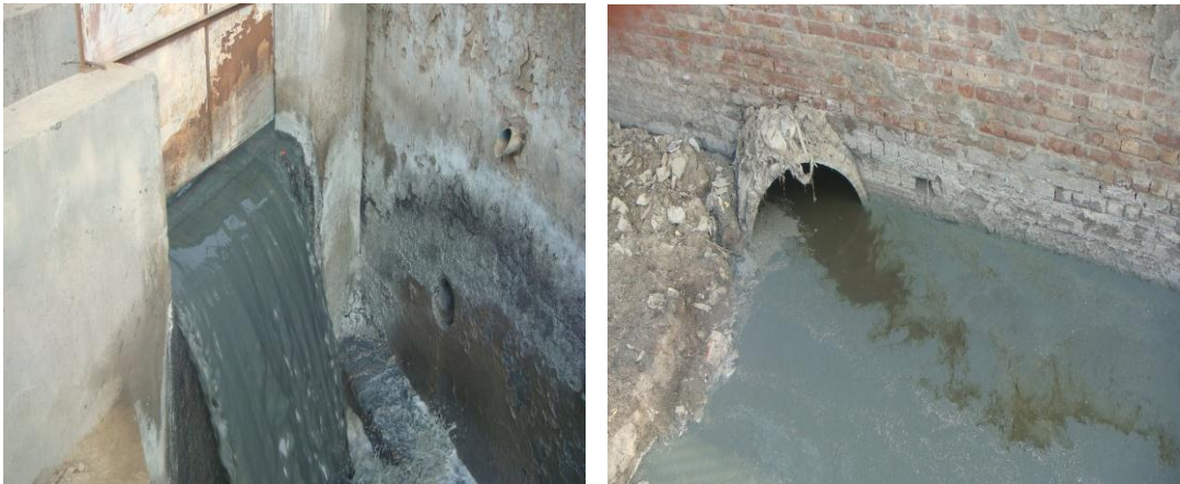
Fig. 4.11: Diversion of untreated effluent and treatment plant effluent in Dec 2009
