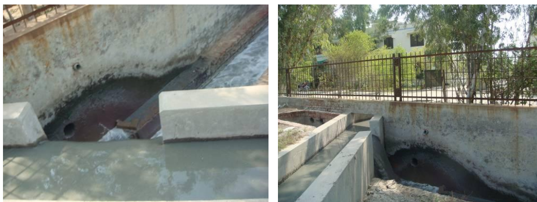
Fig. 4.9: Diversion of untreated effluent before it enters treatment plant (Nov 2008)
