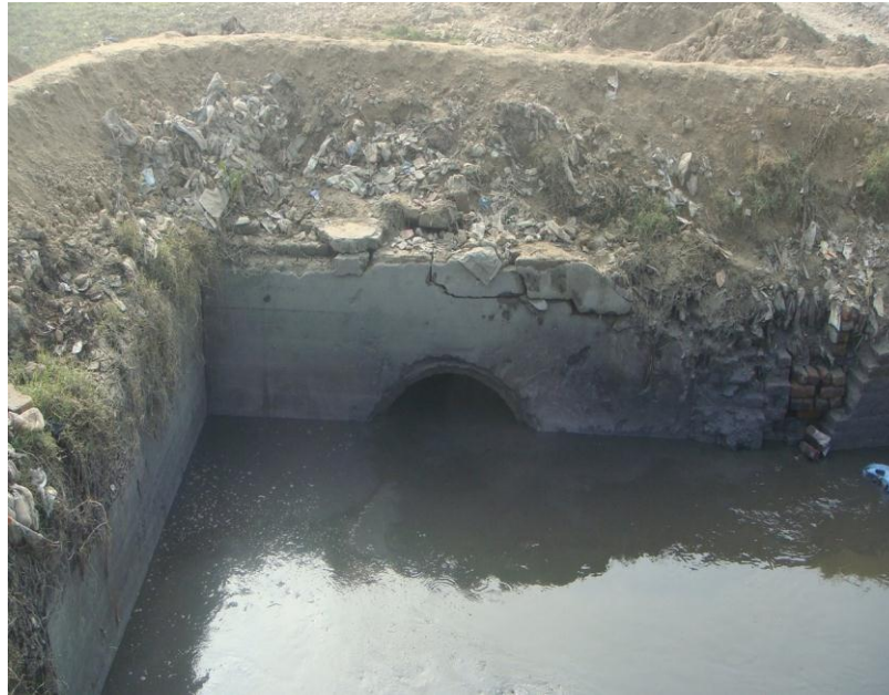
Fig. 4.16: Another view of junction showing the opening point of underground sewer for final disposal into Main Drain (picture taken in Dec 2009)
