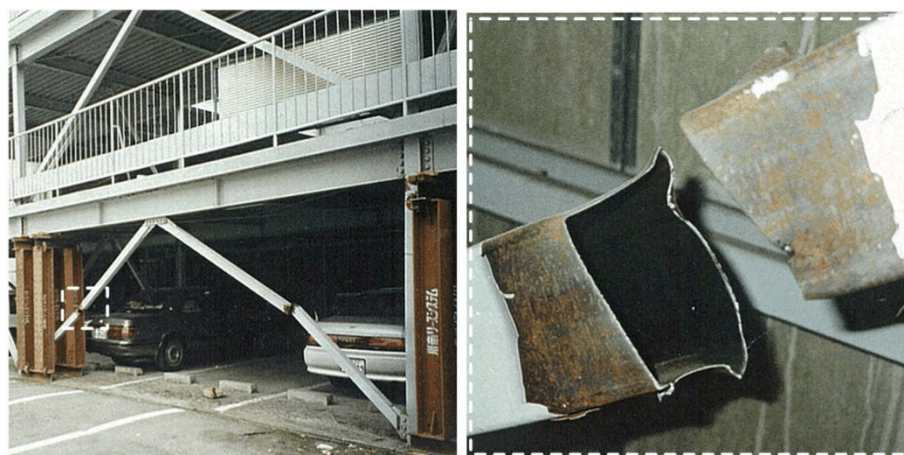
(a) A parking lot in 1995 Hyogoken Nanbu-oki earthquake (Courtesy of Prof. Kuwamura) 1-3)
