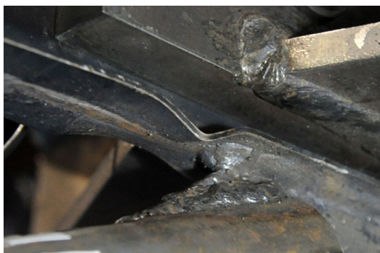
(a) Girder local buckling (150%-2nd, right end)
