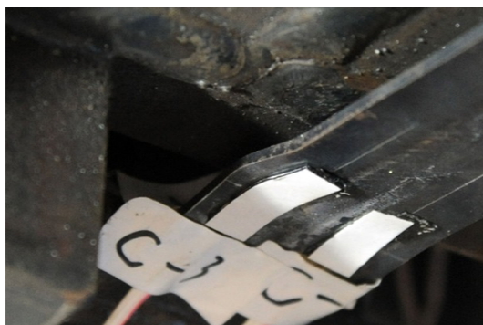
(b) Girder local buckling (150%-2nd, left end)
