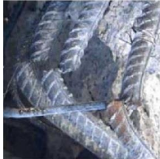
(c) Reinforcement fracture
