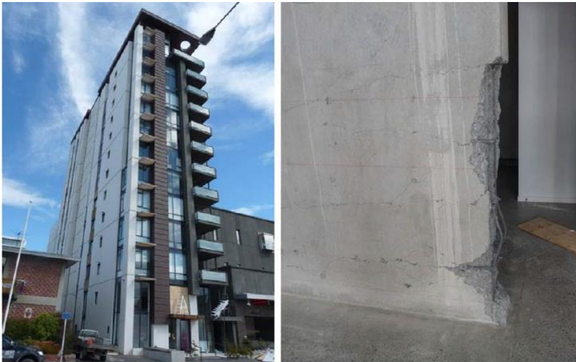
Figure 2.6 - Damage to reinforced concrete structural wall in Christchurch (Credit: Elwood)
