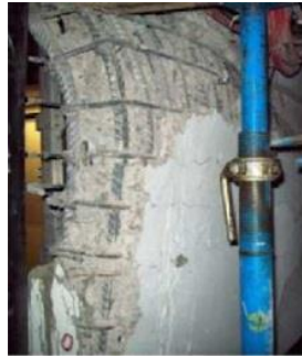
(a) Out-of-plane buckling
